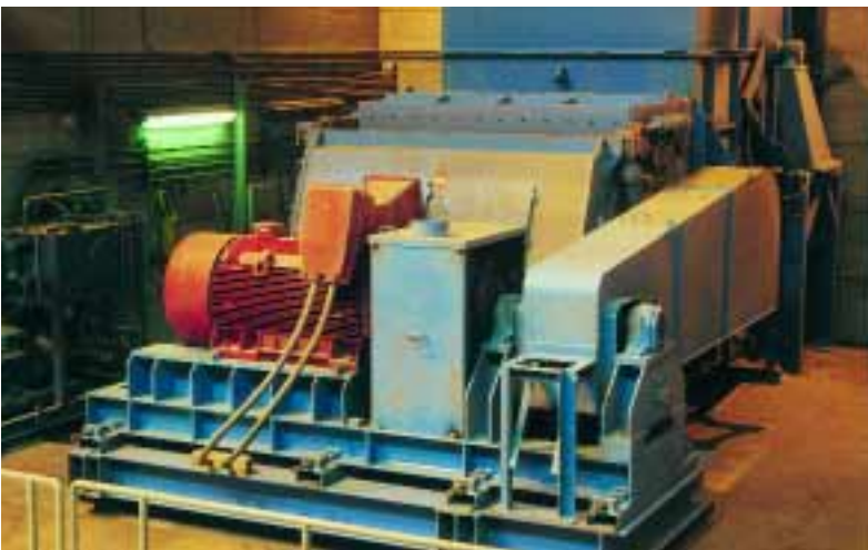
Lindemann KHA 16/24 – 630 kW: plant for recovering fuel from waste, the Netherlands
